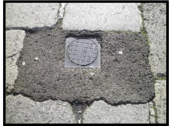
Figures 60 - Use of poor quality materials adjoining historic materials
