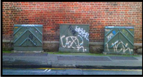
Figure 65 - Corner of North Great Georges Street and Denmark Street Great - prominent junction boxes representing opportunity for innovative street art
