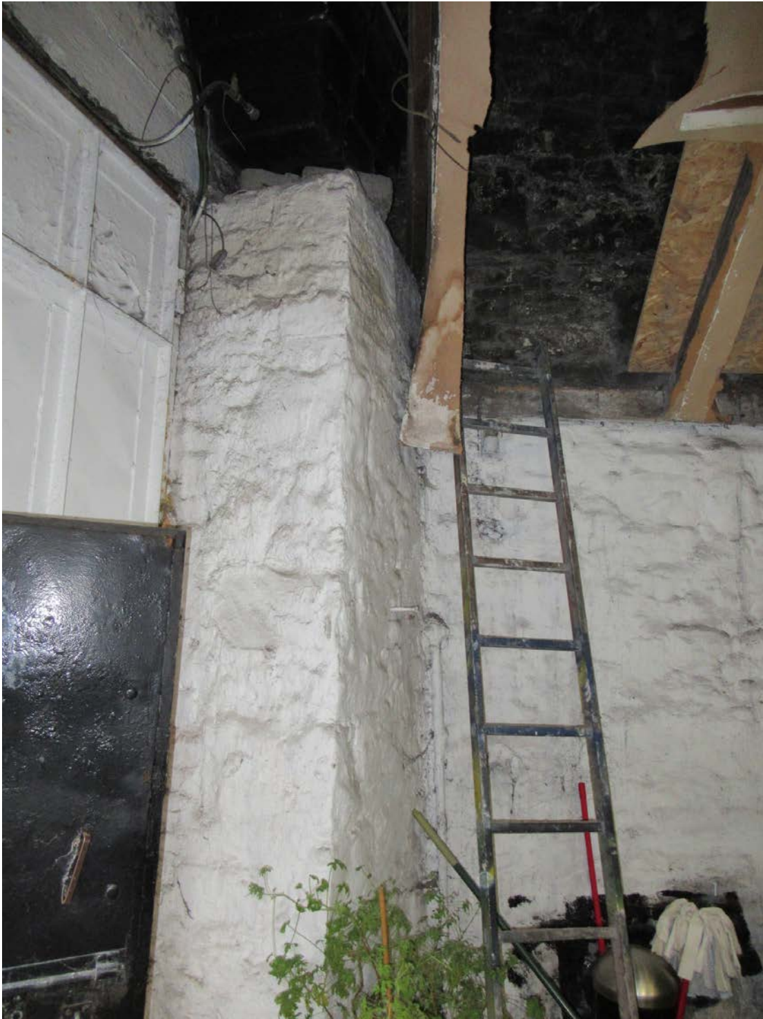
Figure No. 8. Internal detail view showing the rubble stone pier that forms the northeast corner to the current structure at [REDACTED]. This pier also forms the east jamb to the large vehicular gate. The old rubble stone wall behind this pier can be seen to continue across behind this pier to the corner, suggesting that they were not built at the same time.
