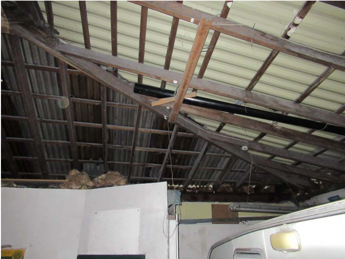
Figure No. 9. Internal view showing the lightweight timber roof structure to [REDACTED], covered with corrugated steel and aluminium sheeting. This roof contains no materials that could date from the C18th or early C19th, and appears to have been built and repaired since the middle of the C20th.
